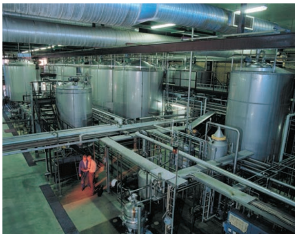
... cooling water systems for power plants, food processing industry, in gas and drinking-water supply lines ...
